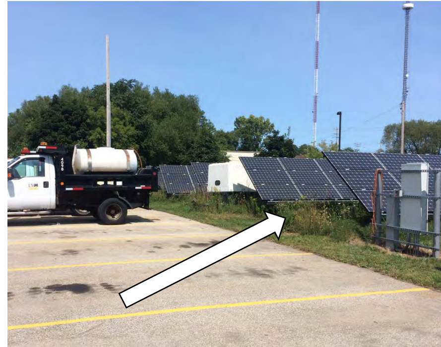
Tall weeds growing in front of some panels
