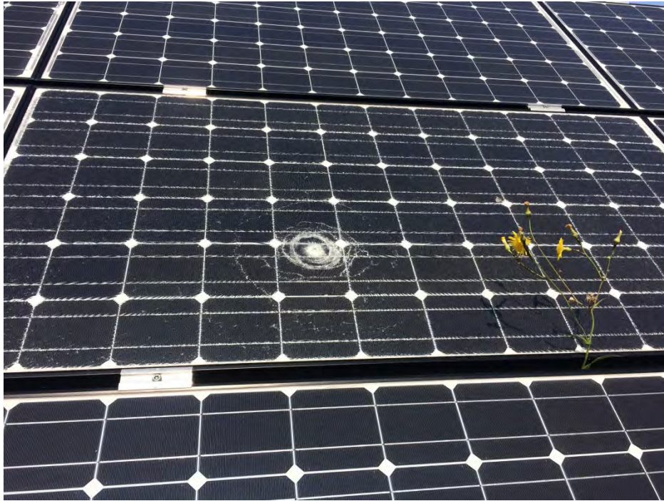
Bullet hole in one of the panels. Cari was able to take students out to test this system.
