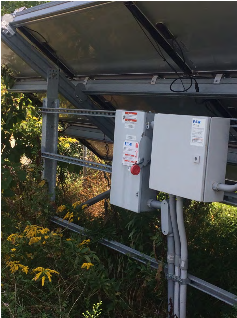
Disconnect switch in 'off' position
